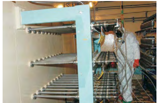
Equipment connected with the In-core thimbles.
