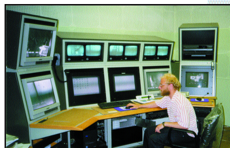
Central alarm stations are used for alarm detection and video assessment.
