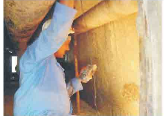
Thickness measurement of Heat Recovery Steam Generator (HRSG) lowerdead spaces at Uch Power Station.
