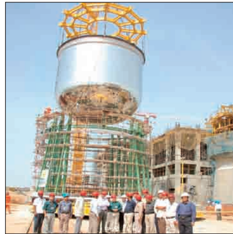
Safety Vessel of PFBR being lifted from Trolley for Erection in Reactor Vault
