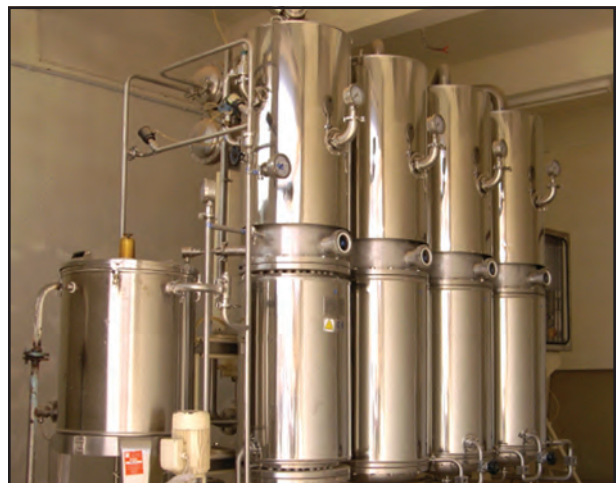
Figure 8. High grade water production plant.
