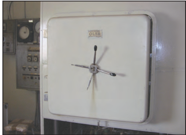
Autoclave with control panel.
