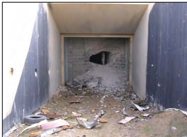
Figure 13. Bricked entryways that were breached.
