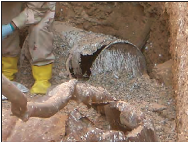
Figure 20. Sloping trenches with exposed drums and debris.
